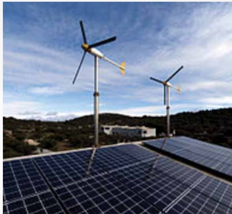
Hybrid System, 2400W, Windturbines , 4000W Solar Modules Zirje Isalnd, Croatia
